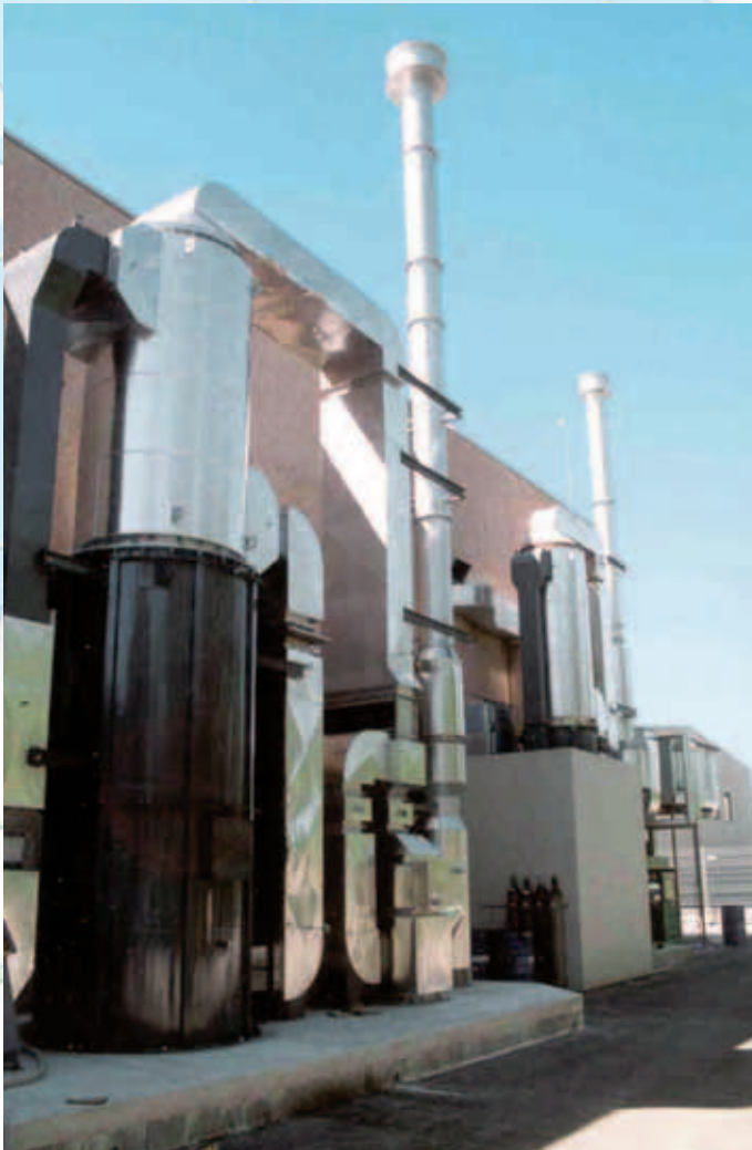
Pharmaceutical Industry • Twin Oxidisers with recovery to air and water • Effluent gas • 6,000 Nm 3 /h
