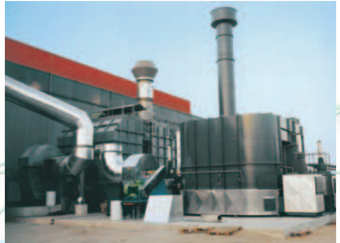
Superficial coils treatment • Twin regenerative oxidisers 45,000 Nm 3 /h installed in different period of times
