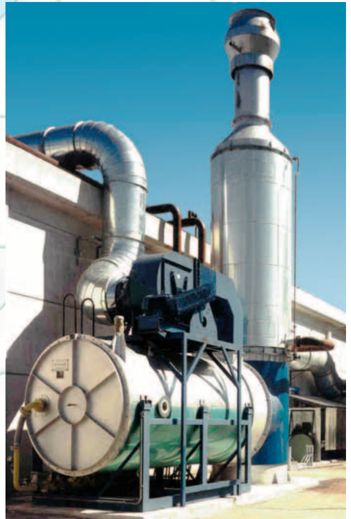
Leather cloth Manufacturing • Effluent gas 20,000 Nm 3 /h • Thermal Fluid Heat Recovery
